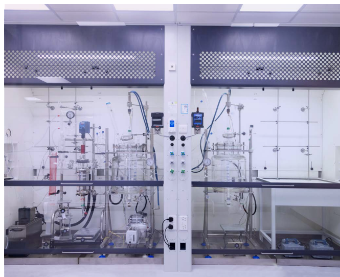
Flexible laboratory design, allowing for less standard activities to be carried out in the same area
